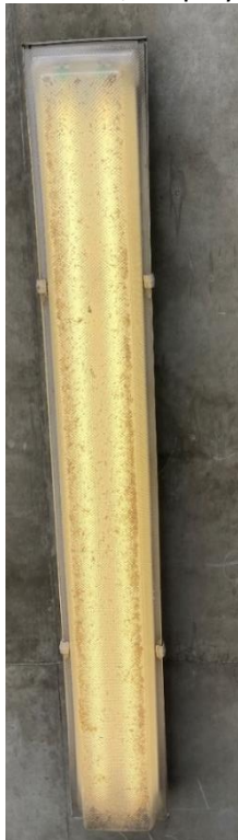
Outside all elevators - fixtures trap dirt & bugs
